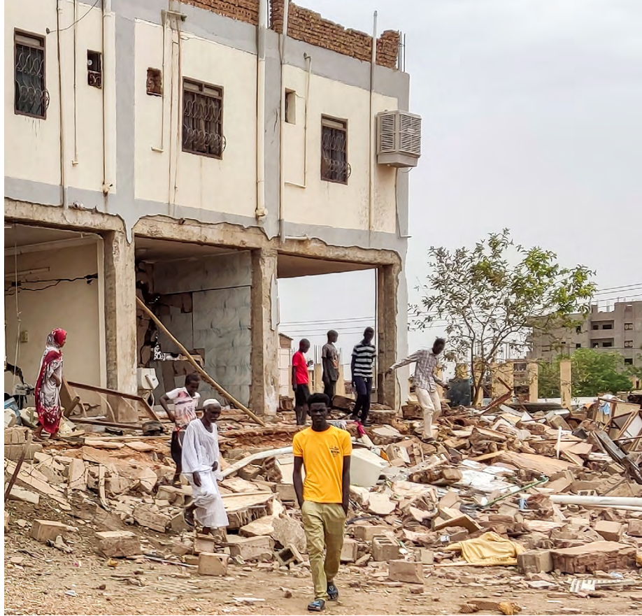
People inspect the remains of a home after it was struck by an artillery shell in the Azhari district in the south of Khartoum.
